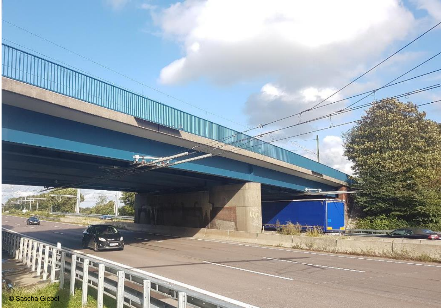
Implementation under a railway bridge with rigid catenary
